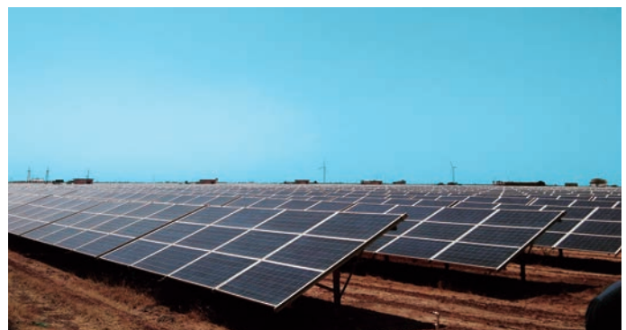
Solar power plant in Gujarat, India. © Prajapati karan v/ Shutterstock
